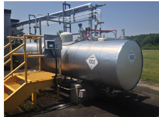
Anhydrous Ammonia Storage Tank
